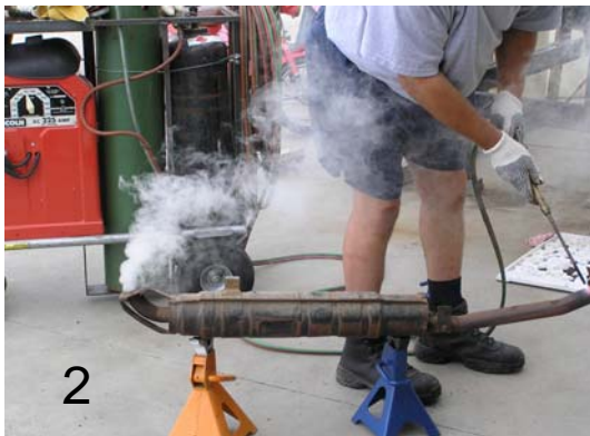
2 Pipe is hot and about ready for air. Big belly guy is also ready for air due to changing wind direction.
